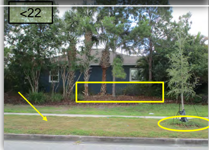
23. Investigated- The zone 12 on controller works properly; Zone 11 valve does not flow properly. Checked the bleeder valve and no water is going through the valve - investigation continuing.
